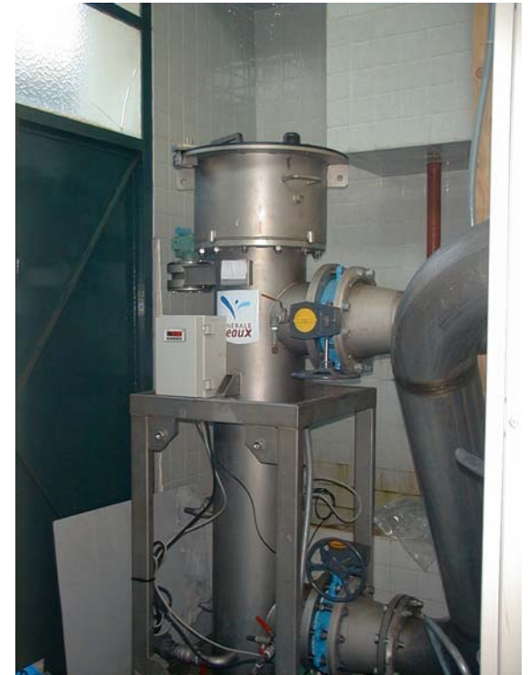
MP-UV installation in Divonne-les-Bains (France)
